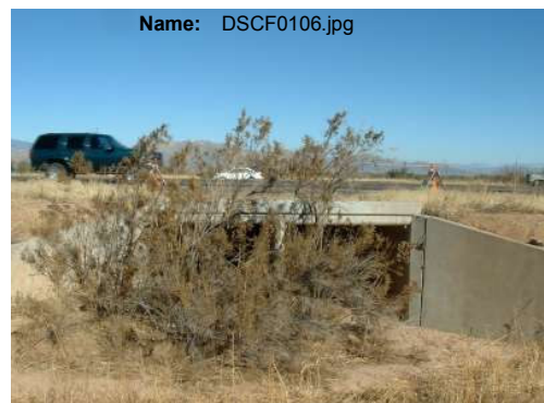
Azimuth: 0 Zoom: 1x Notes: Photo taken from south side of culvert, facing north.
