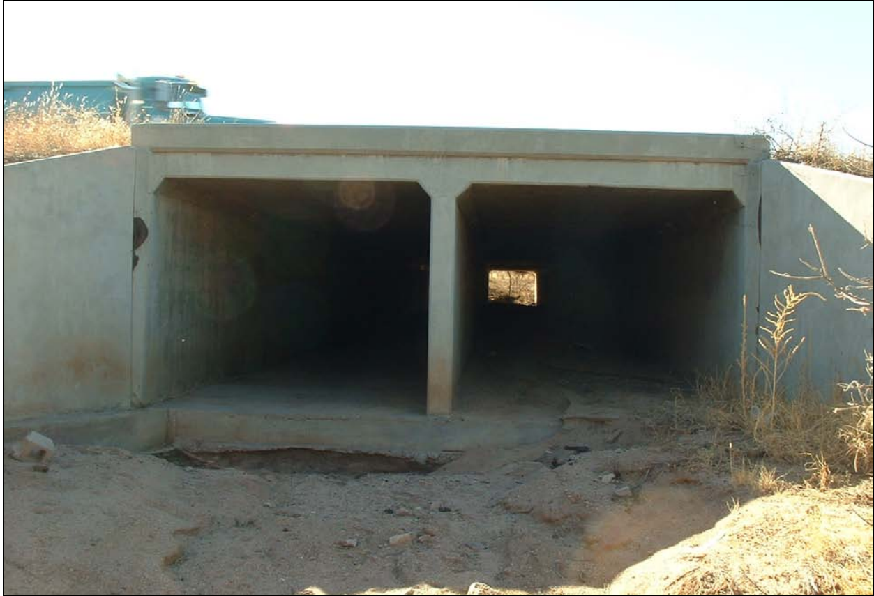
Figure 12: Looking south from waypoint 40, an unnamed wash crosses I-10 in Strand 4 of the linkage design via 2 8x10 ft box culverts. See Figure 5 to locate this scene within the linkage design.
