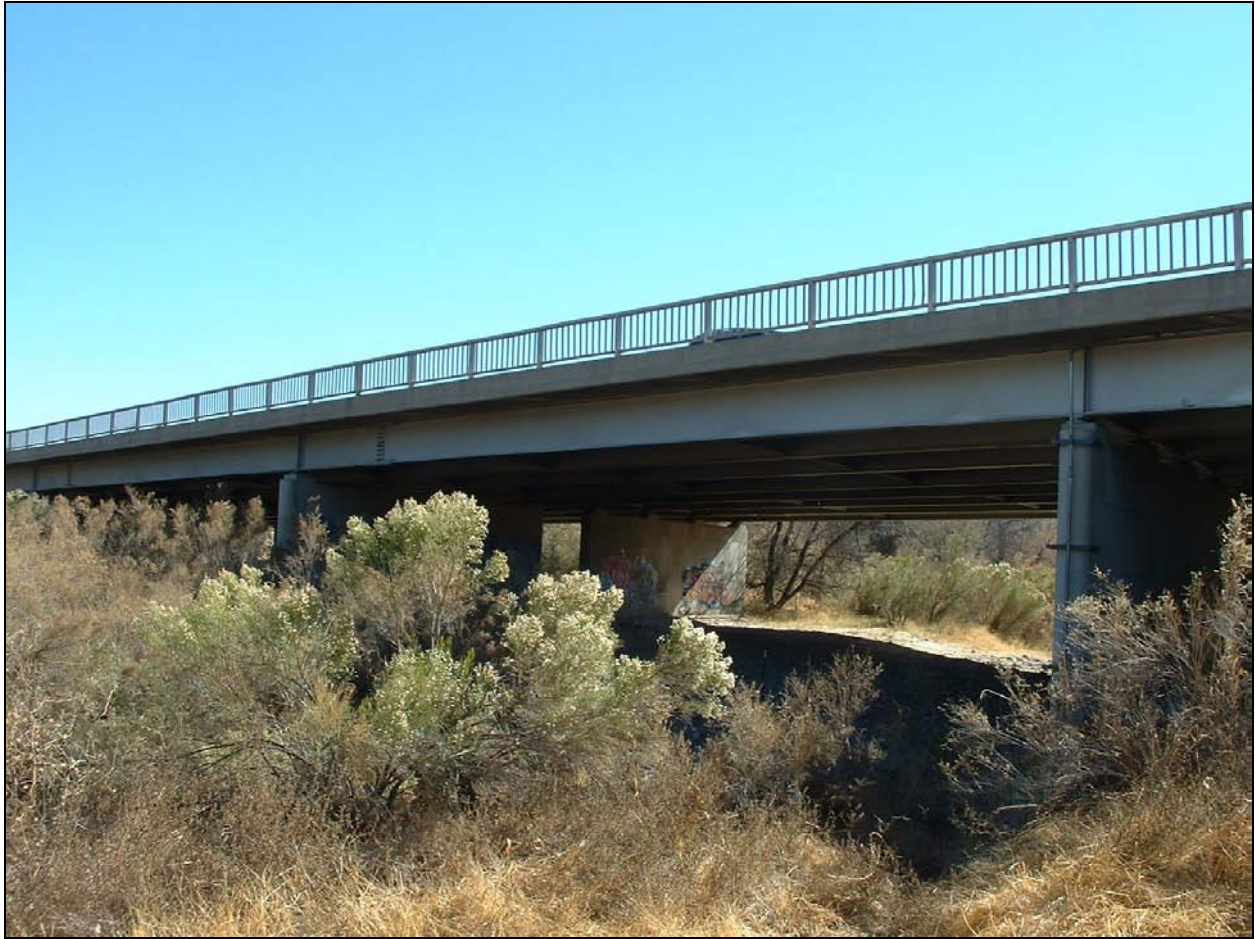
Figure 11: Looking southeast (azimuth 132) from waypoint 49, Cienega Creek crosses I-10 via a large multiple-span bridge. See Figure 5 to locate this scene within the linkage design.
