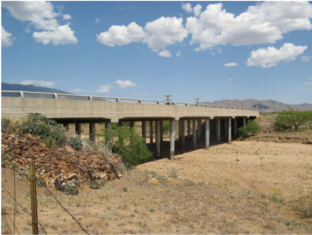
Figure 12: A large bridge along SR 266 near the junction with Klondike Rd, Waypoint 66
