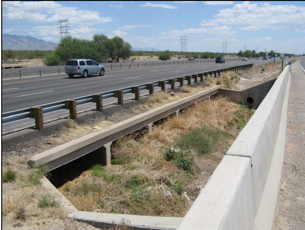
Figure 14: Six 24" box culverts under I-10 at Waypoint 26, blocked by brush.
